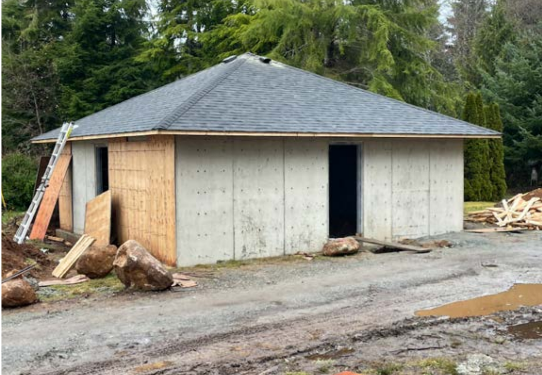
Construction of Alert Bay campground facility Source: Village of Alert Bay and B.C. Ministry of Tourism, Arts, Culture and Sport
