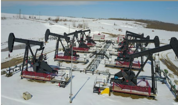
Exhibit 3: Site producing natural gas condensate with multi-well pad and associated piping and facility in northeastern B.C.
