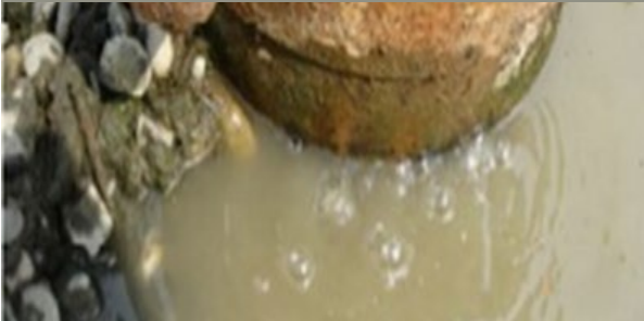
Exhibit 12: Gas bubbling up at a wellhead from a leak
