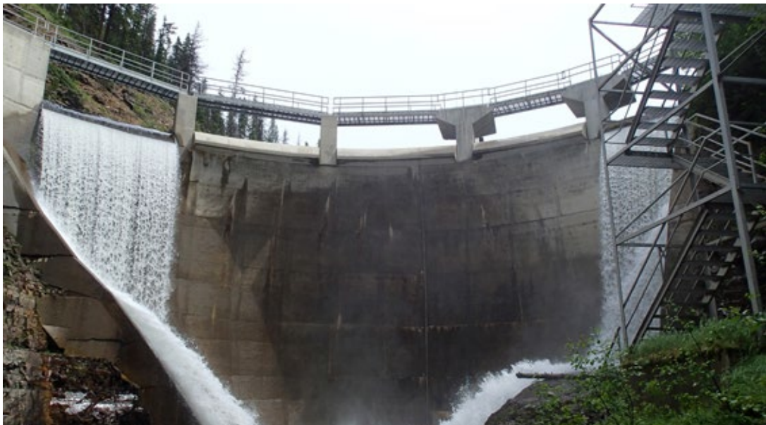
Mark Creek Dam in the Kootenay Region (extreme-consequence dam). Photo credit: Ministry of Forests, Lands, Natural Resource Operations and Rural Development
