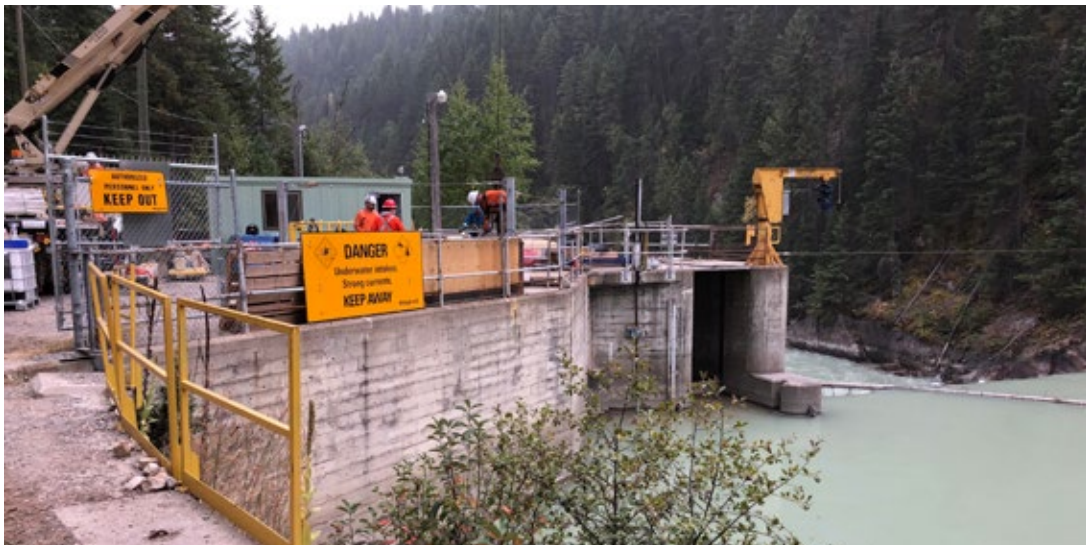
Spillimacheen Dam in the Kootenay Region (significant-consequence dam). Photo credit: Ministry of Forests, Lands, Natural Resource Operations and Rural Development
